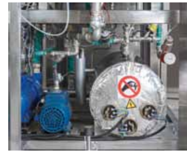
Integrated Steam Generator with Water Supply Pump
