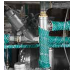
AISI 304 Stainless Steel Piping with Heat Insulation
